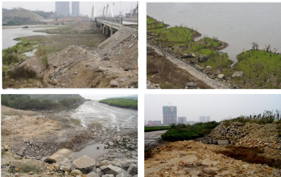
Figure 2 Existing Problems Before Ecological Improvement in Xiwan Hongshahuan. Top-left: Exposed seawall. Top-right: Eroded mudflats. Bottom-left: Urban sewage outlet. Bottom-right: Exposed mudflats and shoreline. (Wang Xin, 2012)
